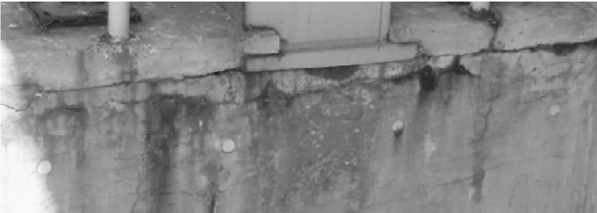
Dark spots and streaks show internal rust on the old stairway (currently the up side steps).
