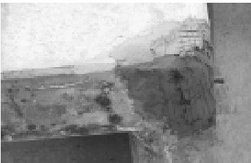
Behind the Manhattan Tramway station, looking up near the new stairway reveals this remade corner, patching a spall. Dark spots nearby are additional spalling.
