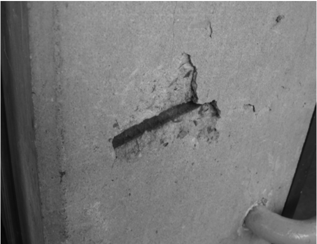
Spalling occurs when rusting rebar forces concrete to fall away. It’s one of many non-safety problems cited by RIOC’s Tramway consulting team. This example is at the Manhattan station, on the platform.
